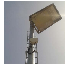
RTMS Sx-300 unit installed with a solar panel on the side of the highway.
